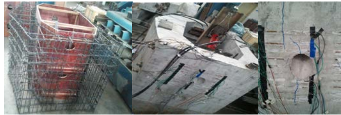
(a) Assembling reinforcement (b) concrete placement (c) crack distribution Figure.4 Scale model experiments
