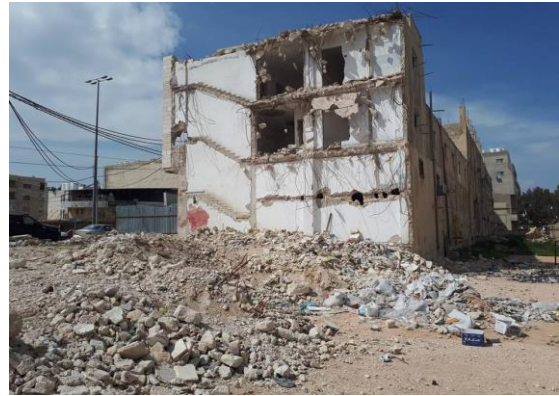
Figure 1. The demolishing of some buildings in Irbid City during requalification process. (Source: Author, 2019)
