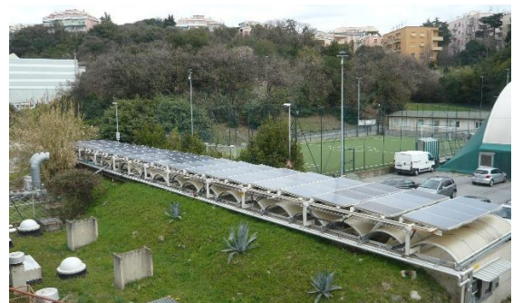
Figure 3. Solar field of Palacus plant
