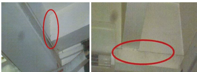
Figure 10: Results of damage assessment – building 1.
