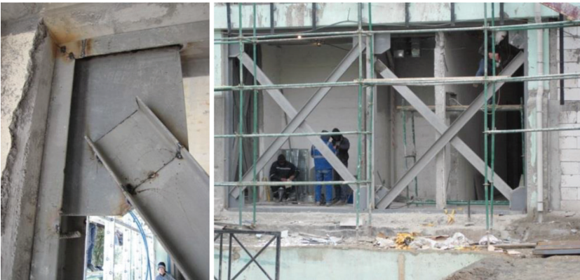
Figure 7: Unplanned use of steel bracings.
