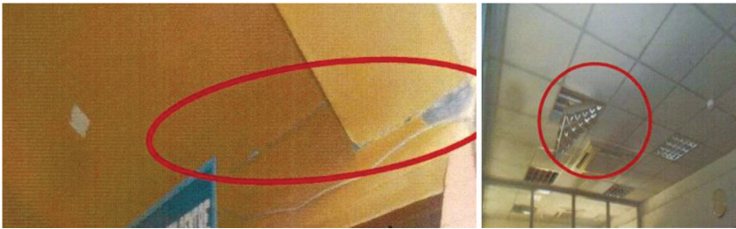
Figure 11: Results of damage assessment – building 2.
