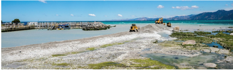
Figure 7: Repair to the Kaikoura Harbour, which rose 1–2 m during the earthquake – emergency works are occurring under section 330 of the RMA. (Source: T Madsen, Feb 2017).
