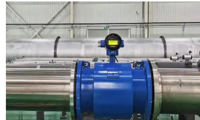
Figure 2. Electromagnetic flowmeter on the pump pipeline
