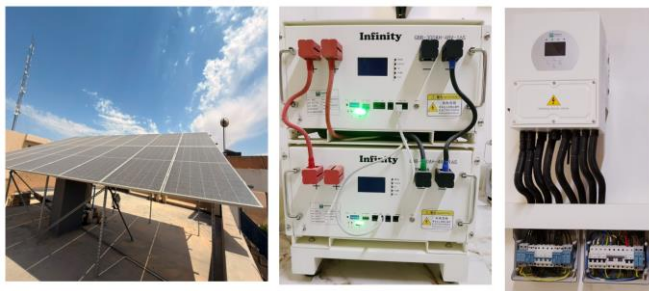
Figure 2. Experimental hardware components including the 16 Photovoltaic (PV) modules, storage batteries, and hybrid inverter
