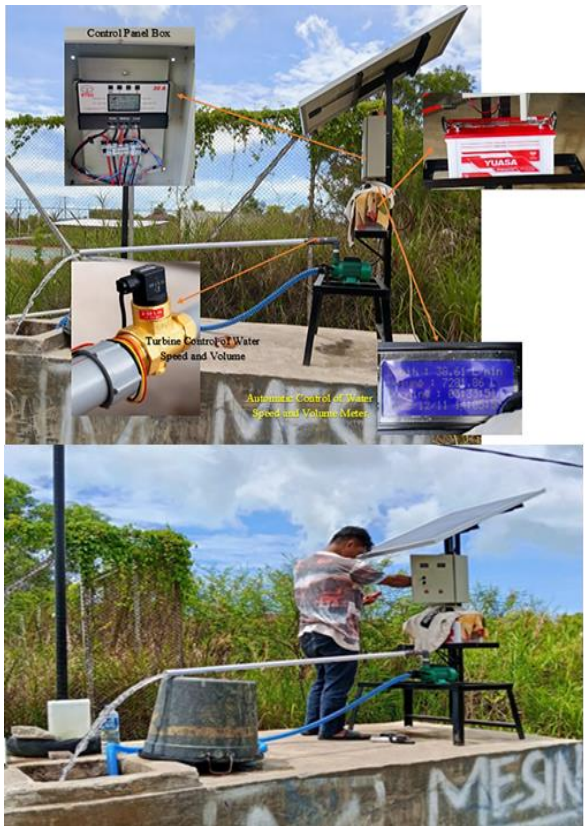
Figure 1. Solar powered irrigation pump system
