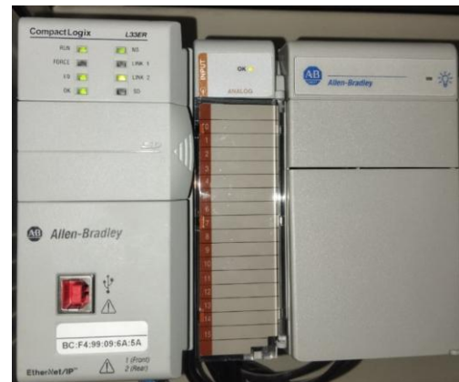
Figure 5. Allen-Bradley 1769-L33ER CompactLogix Programmable Logic Controller (PLC)
