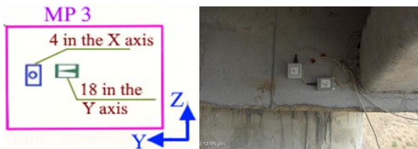
Figure 6. Accelerometers located at observation point 3
