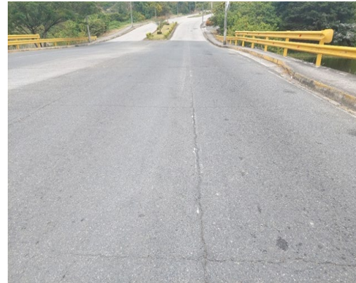
Figure 14. Slab joints and distress reflected on the asphalt overlay (station 1+040)
