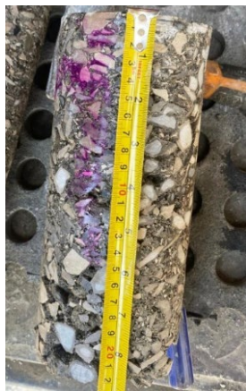
Figure 12. Voids in concrete core (station 1+460)
