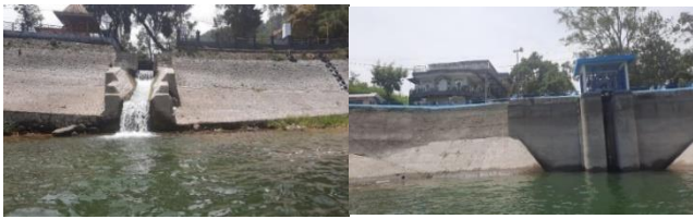
Figure 2. Location of net installation and water quality observations inlet (left) and outlet (right)
