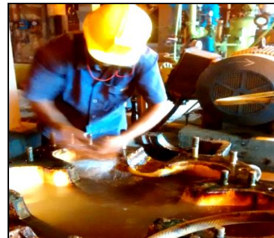
(a) Pump Internals and Pump impeller
