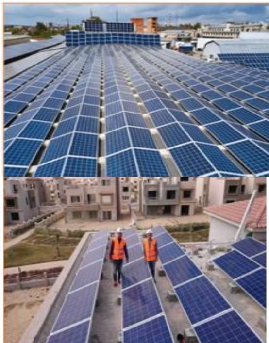
Figure 14. Integration of solar cells on a building roof [31]
