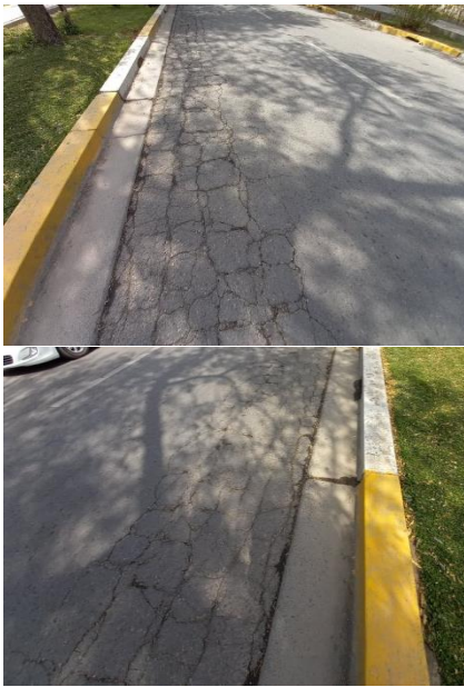
Figure 1. The alligator cracks on the side of the University of Baghdad campus road
