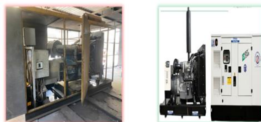
Figure 1. Perkins deiseal generator
