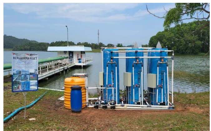
Figure 2. Actual picture of U-type membrane ultrafiltration system installation
