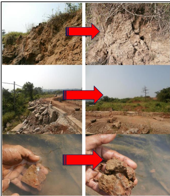
Figure 4. The typical existing condition of slope at the Cisadane watershed and / or river basin and fine-grained soil collapse during the rainy season every year
