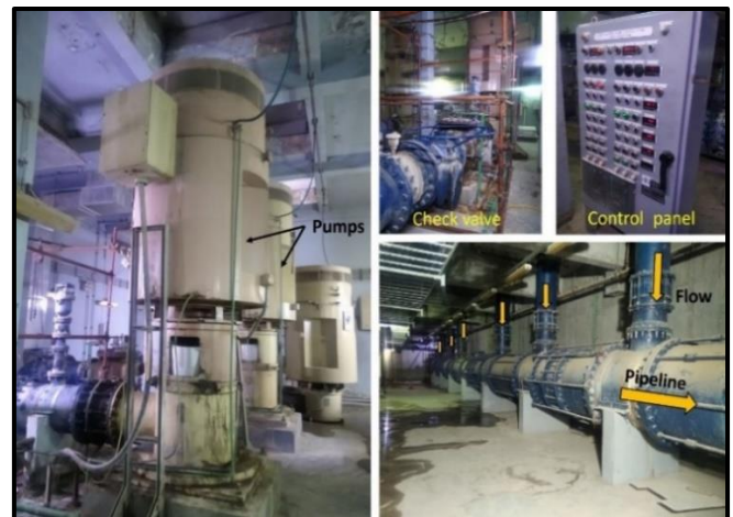
Figure 10. The pump station, pipeline, and control panel at the main pumping station
