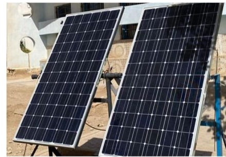
Figure 3. Photovoltaic panels utilised in this study
