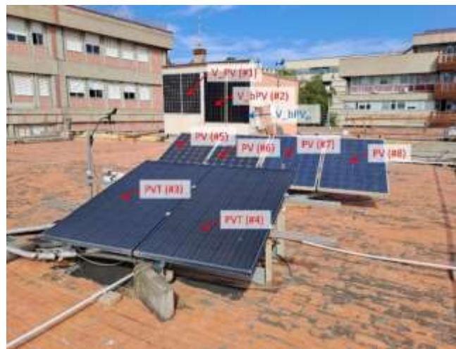
Figure 3. Layout of monitored PV plant
