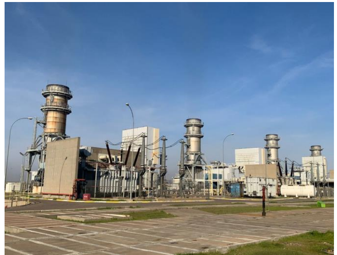
Figure 3. Qayyarah gas power station [7]
