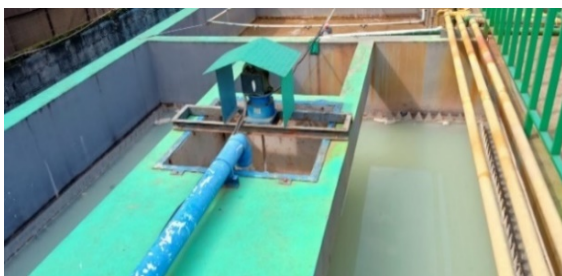
Figure 4. Primary settling tank
