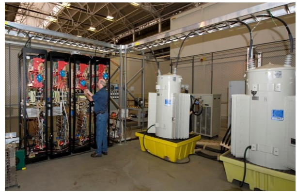
Figure 3. General Electric prototype comparison between solid-state transformer and traditional one [24]
