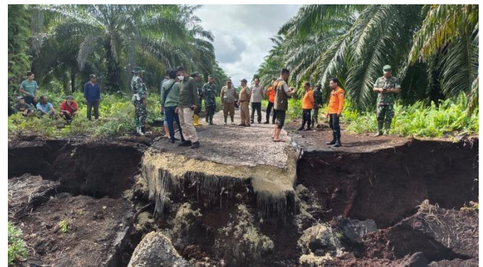
Figure 2. Abrasion on Bengkalis Island resulted in damage to infrastructure such as roads
