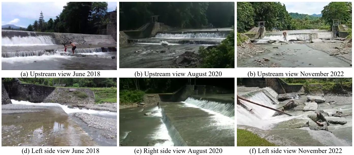
Figure 2. Condition of stilling basin of Sibado Weir 1998-2022
