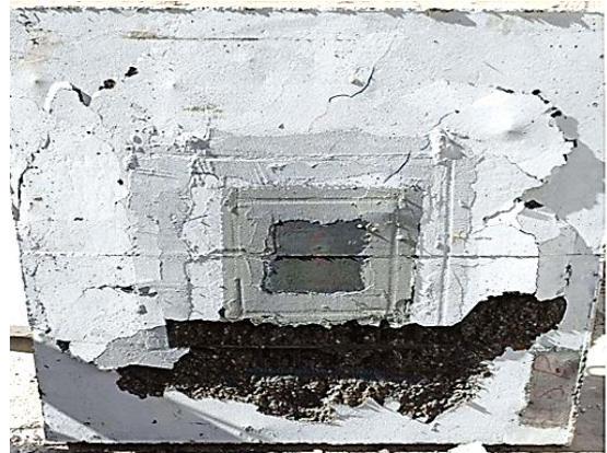
Figure 14. Crack pattern of slab (HSB) at failure
