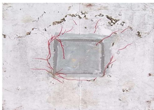
Figure 6. Crack pattern of slab (NSB) at failure
