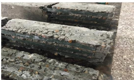
Figure 4. Splitting of cover due to high quantity of reinforcement
