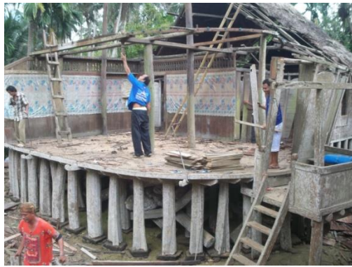
Figure 4. A traditional house damaged by the earthquake is in the process of being rehabilitated
