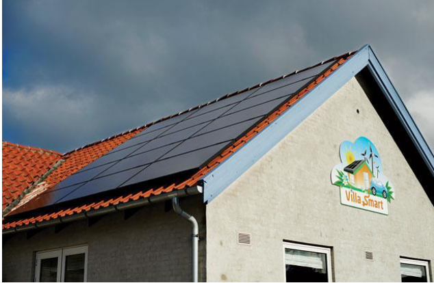
Figure 6. Photovoltaic installations in public housing
