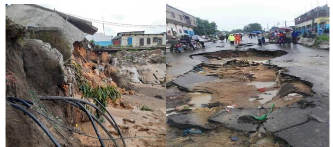
Figure 7. Damage to urban networks Source: Attipo December 2019
