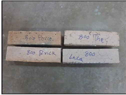
Figure 9. The Cracks on the Surface of Geo-Polymer after exposed to 800°C (Own source)
