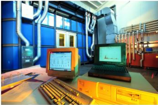
Figure 2. Monitoring and control unit
