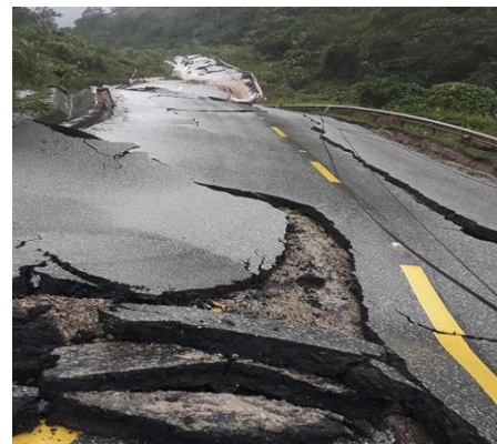
Figure 1. Damage to road as a result of landslide (Image posted by VNExpress)
