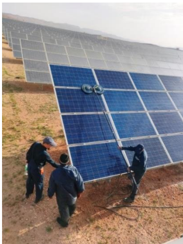
Figure 17. Photograph of dust accumulation clean-up operation
