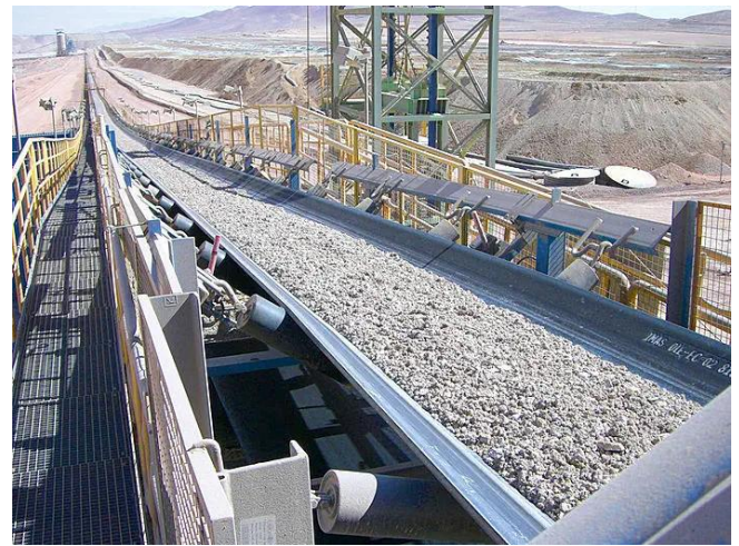
Figure 2. Belt Conveyor in Bir El Ater Mine, Algeria
