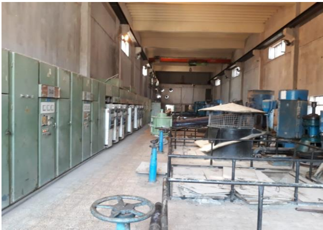
Figure 1. Pump house of Dora SPS
