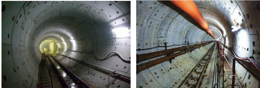
Figure 1. Interferences on tunnel surface
