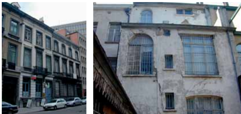
Figure 3: Front and back façade of the renewable energy house, Brussels, before refurbishment. Source: Adapted from New4Old [27].
