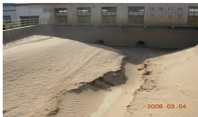
Figure 1. Typical conditions of sediment in forebay
